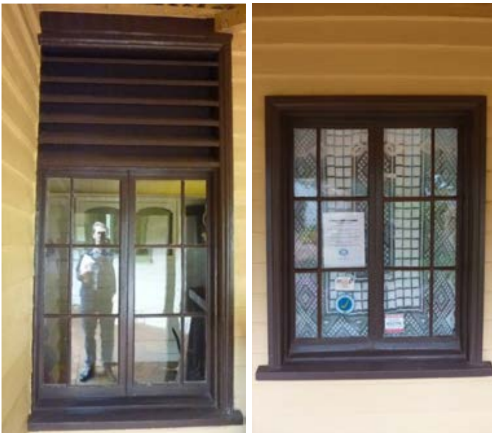
Figure 49 Early casement windows on the south-west elevation of the house: the window at the north-west end of the elevation (left), is an early form of ventilation
